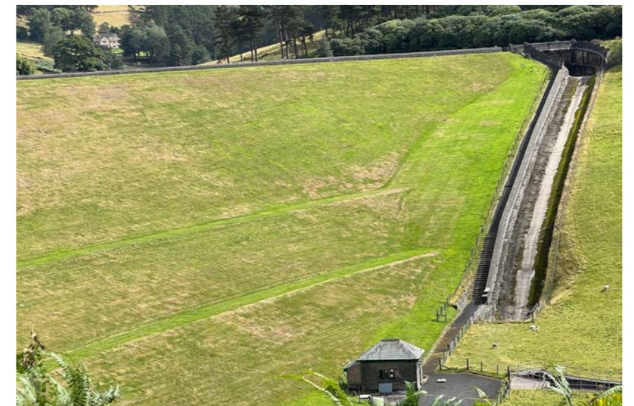
Example of one of the ways that a spillway can be designed, Kinder Reservoir.
