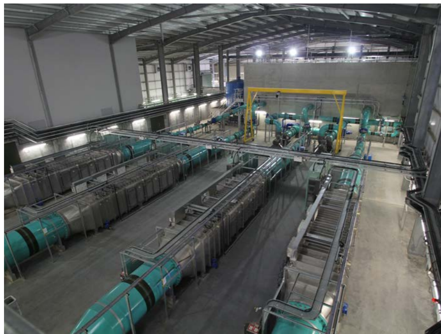
Hall Water Treatment Works
